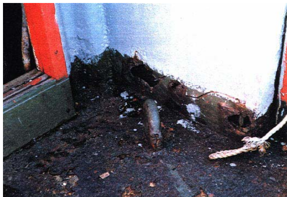
Photograph 1 Corroded accommodation house side structure
